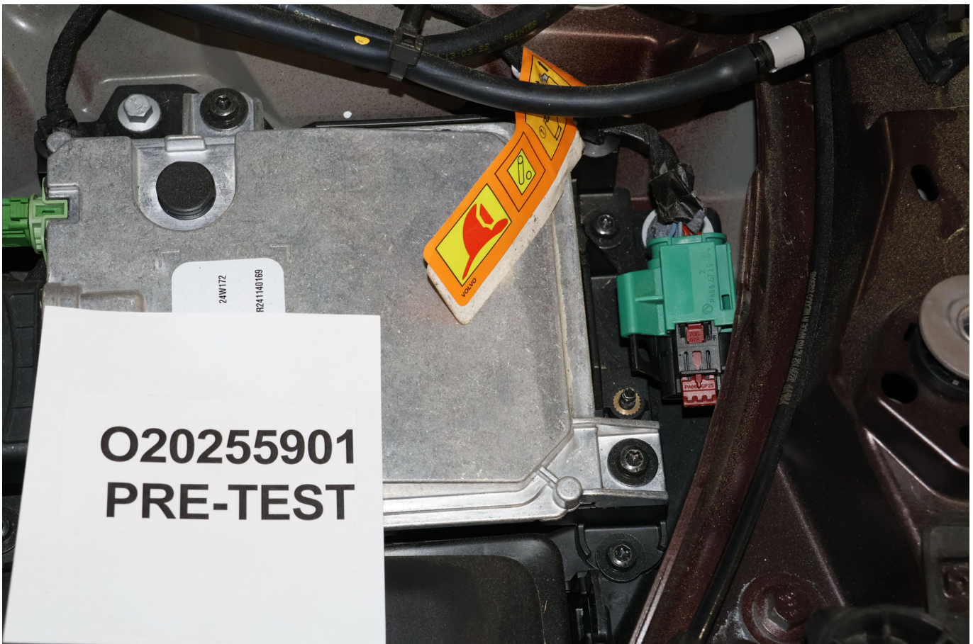
Photo No. 305-03 - First Responder Warning Label
